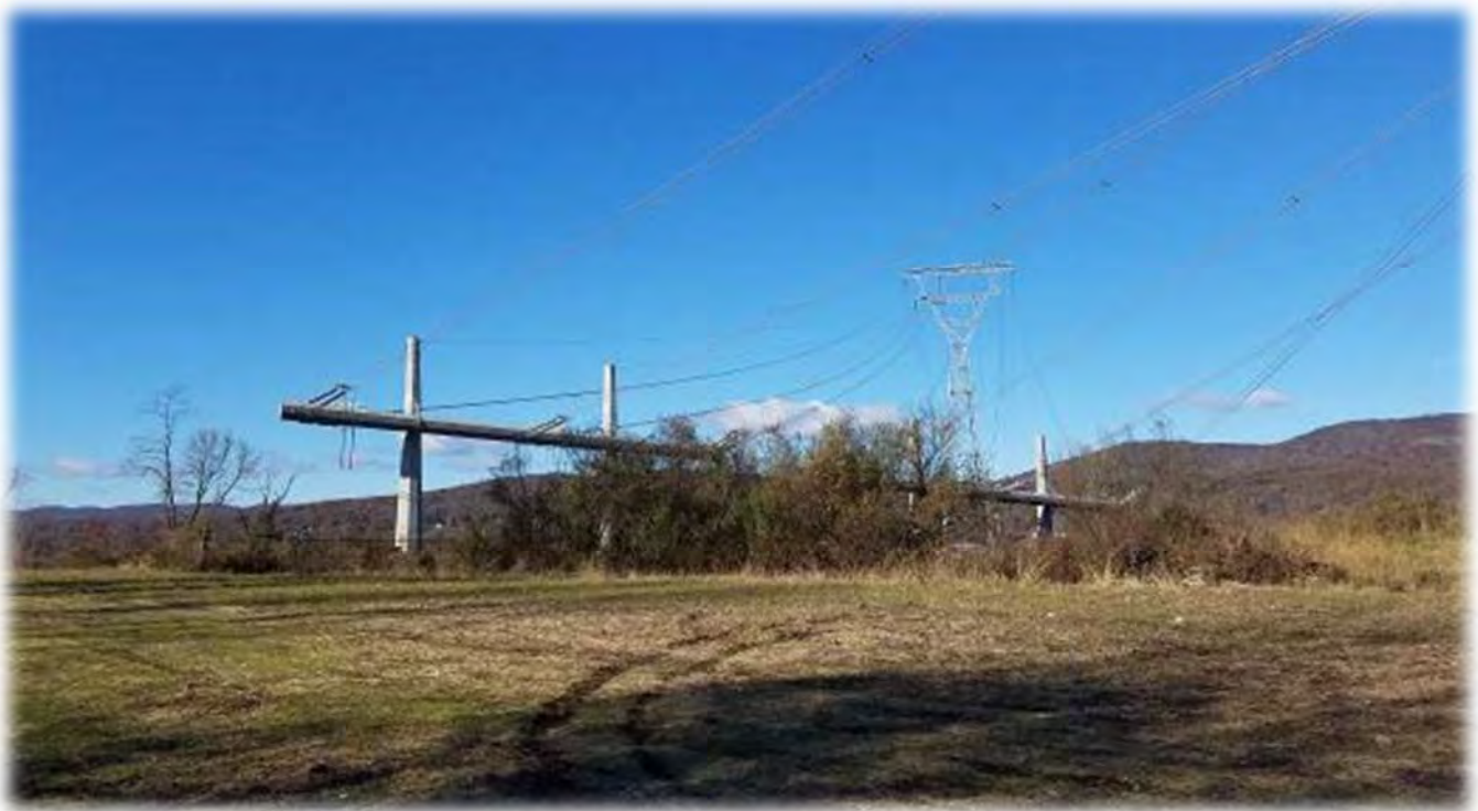
Photo of Con Edison Infrastructure (Retained Parcel #2)
